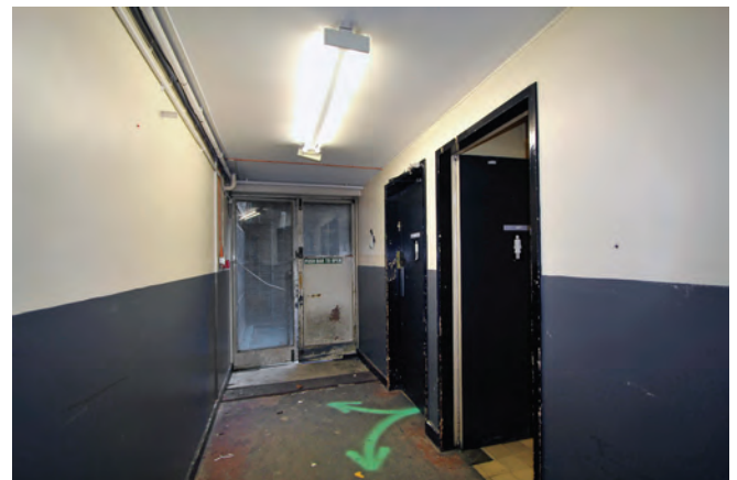
One access to the Emergency Centre spine corridor is down a ramp at the rear of the building. Blast doors were never fitted with just an ordinary door offering little protection
